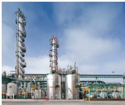
Carbon capture and storage (CCS) plant in Brindisi, Italy © Enel Sharing
